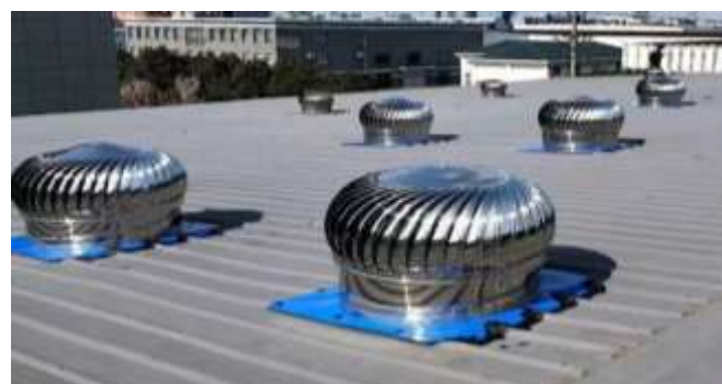
Figure 3. Turbin Ventilator in The Warehouse Rooftop (Source: hbjinbang.en.made-in-china.com, 2022)
