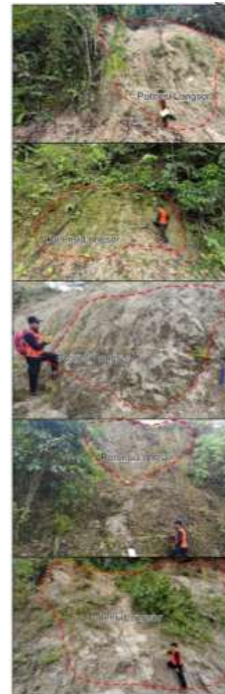
Figure 7. Appearance of slope conditions and landslide potential at stations 1, 2, 3, 4 and 5 (in order from top)
