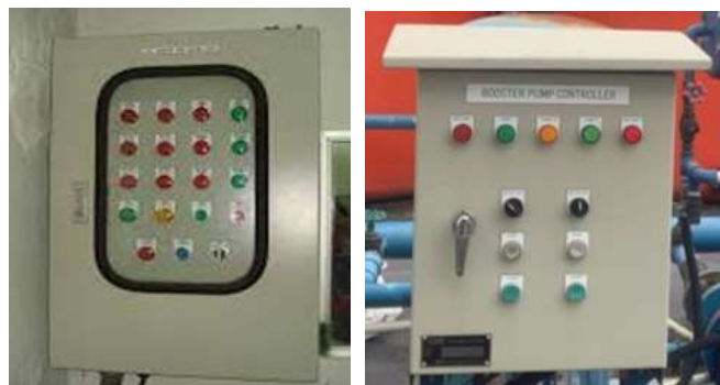
Figure 7. Transfer pump controller and booster pump controller
