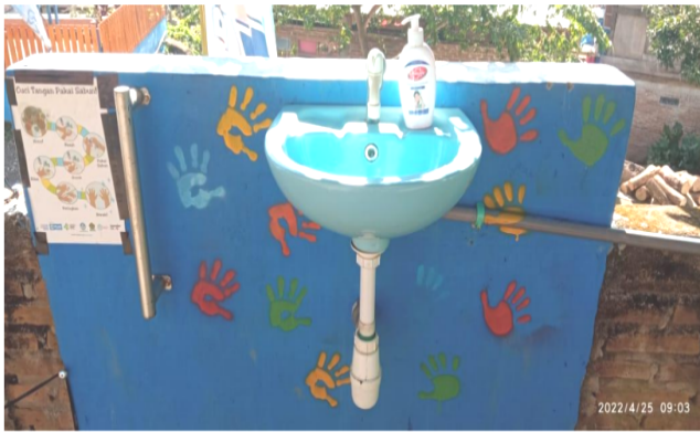
Figure 2. Handwashing facilities at SD Negeri Batudulang, Kab. Sumbawa
