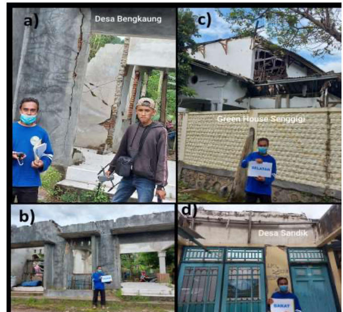
Figure 1. Damage photos: a) and b) in Bangkaung Village, c) in Senggigi (Northwest of Bengkaung), d) in Sandik Village (South Bengkaung) (Hyodo et al., 1993)
